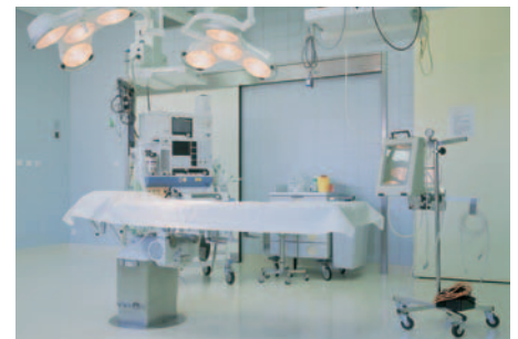
Negative pressure helps prevent the spread of germs and dust particles in hospitals and research laboratories, positive pressure secures operating theatres.
