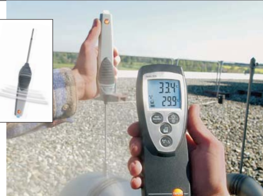
Monitoring temperature at exhaust outlets
